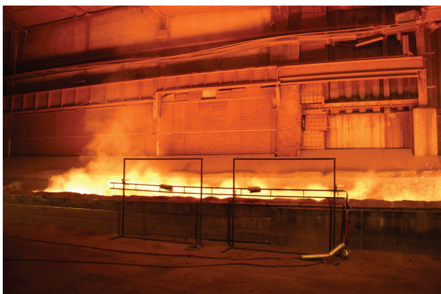
Figure 11: Fine mist sprayers installed at bed top surface level
