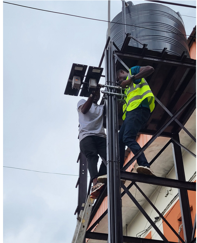
Figure 2: Installation of low-cost monitors in the campus of the University of Douala, Cameroon (credit: LCS-WACA project)
